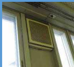
窓設置の換気扇
